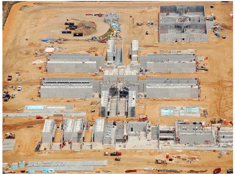
BLACKWATER RIVER CORRECTIONAL FACILITY July 27, 2009 Segregation/Support, H1, H2 & H5 Viewed Looking East
